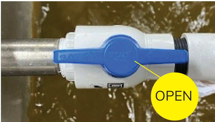
Sump Drain Valve (Open)
