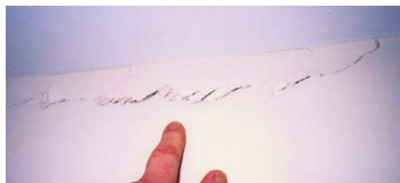
Figure 4: Crack caused by shear.
