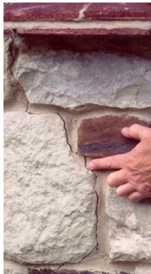
Figure 13. This crack is aesthetic damage only.
