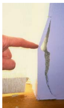
Figure 5: Crack caused by compression.
